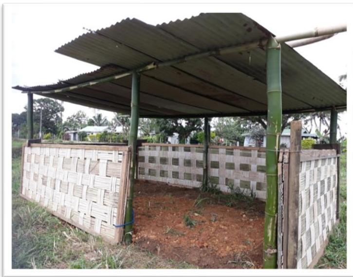
A calf shed made from locally-available materials, such as bamboo and second-hand tin. Using treated pine posts for each of the four corners will make this shed last longer.
