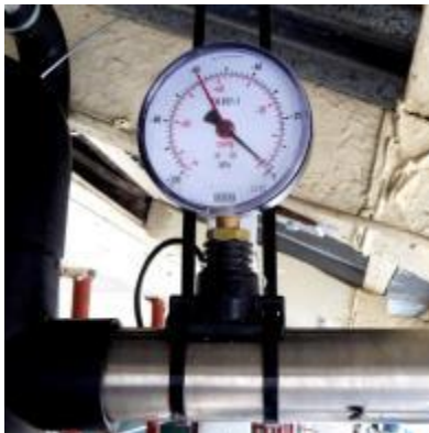
A gauge to check the vacuum level.
