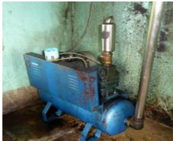
Pump and motor mounted on interceptor/vacuum tank to protect vacuum pump from damage.
